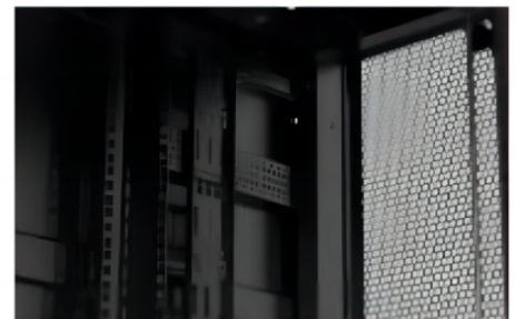
Cable management rails in rear
